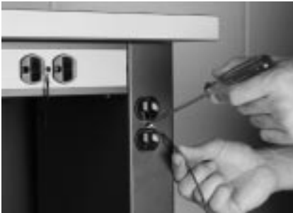
Fig. 7A - Attaching system grounds. Note work surface and unit are grounded at different locations.
